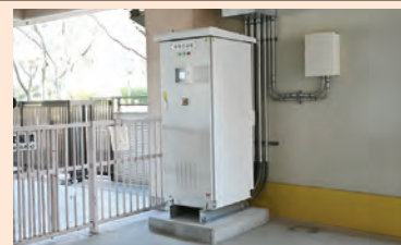
蓄電池 Storage Batteries
